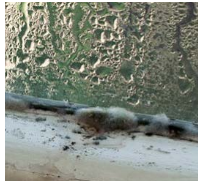
Figure 2 - Mould growth from window condensation
