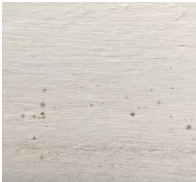
Figure 1 - Mould growth at target site
